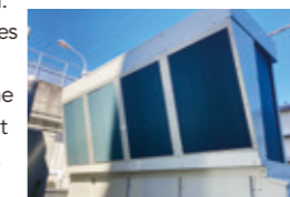
Equipment at the Soka Factory that uses a new refrigerant
